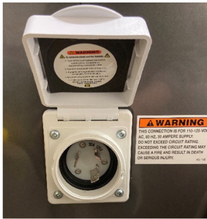
Exterior RV Style Electrical Cord Hook-Up
