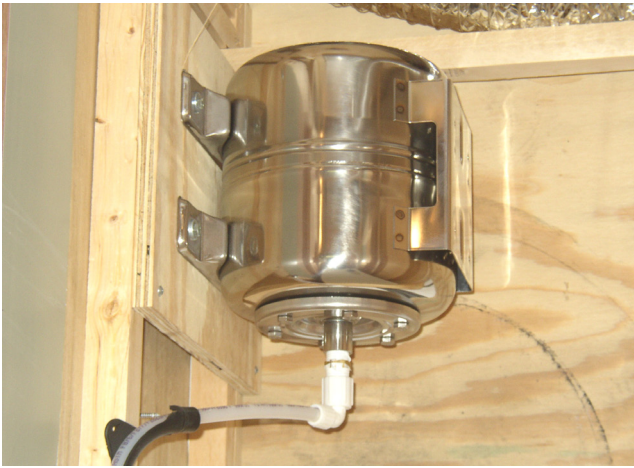
Accumulation Tank (Mechanical Room)
